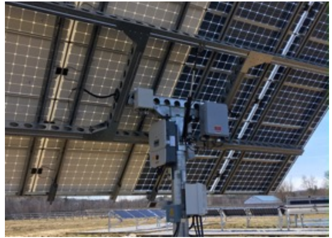
Fig. 16. Backside of Tracker One, with DC monitoring box and datalogger mounted on the pedestal. Monofacial modules are on the left side; bifacials on the right. Backside shading proved to have minimal impact on the bifacial gain for this system.
